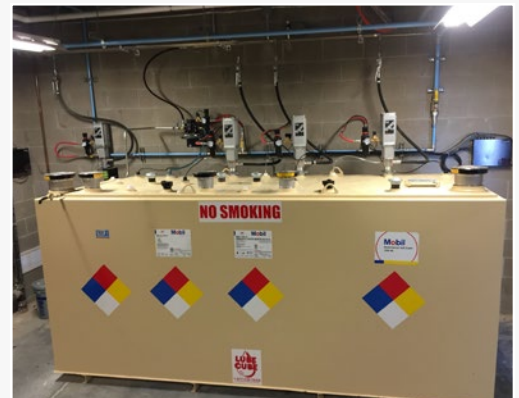
1,250 gallon, 4 compartment tank.
